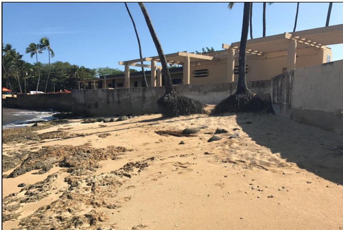
Figure 16. Beach in Front of Seawall and Comfort Station
