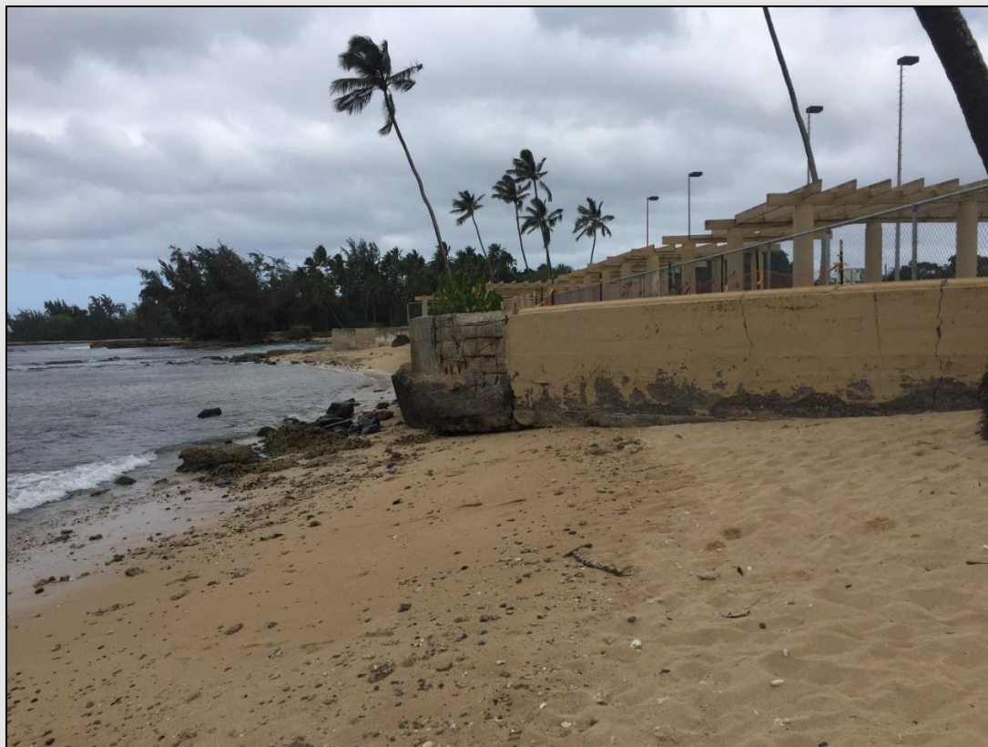
Figure 18: Hale‘iwa Beach Park Erosion
