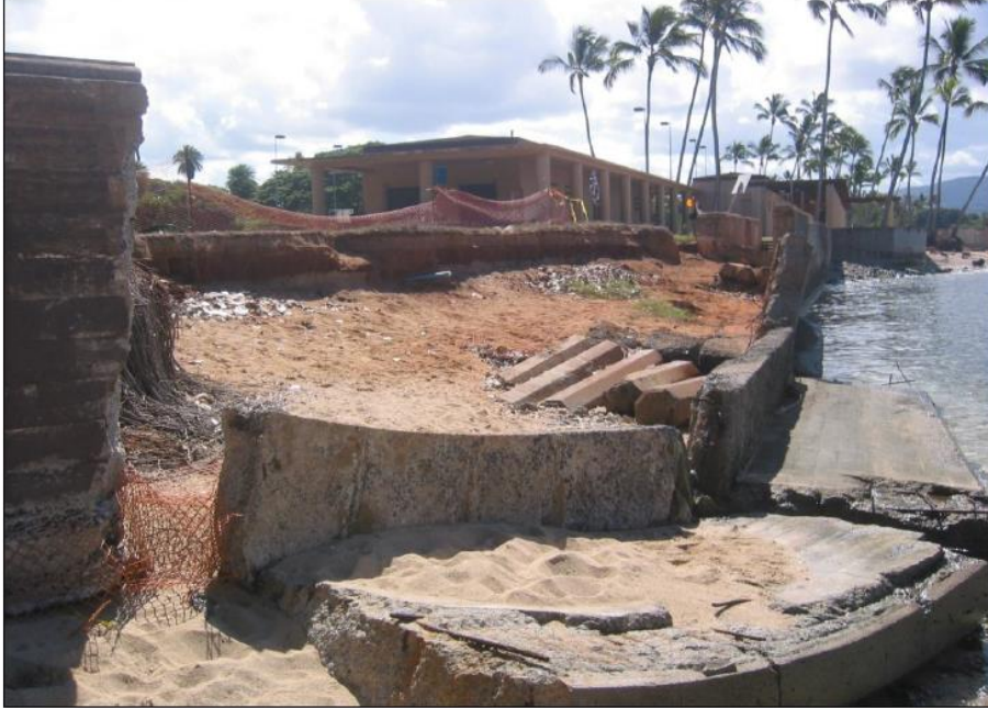
Figure 2-17 Damaged north end of wall (2008)
