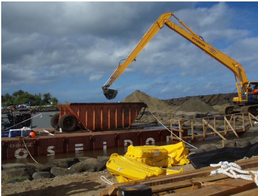
Figure A20. Typical method of mechanical dredging at Hale‘iwa Harbor (from 2009 construction)
